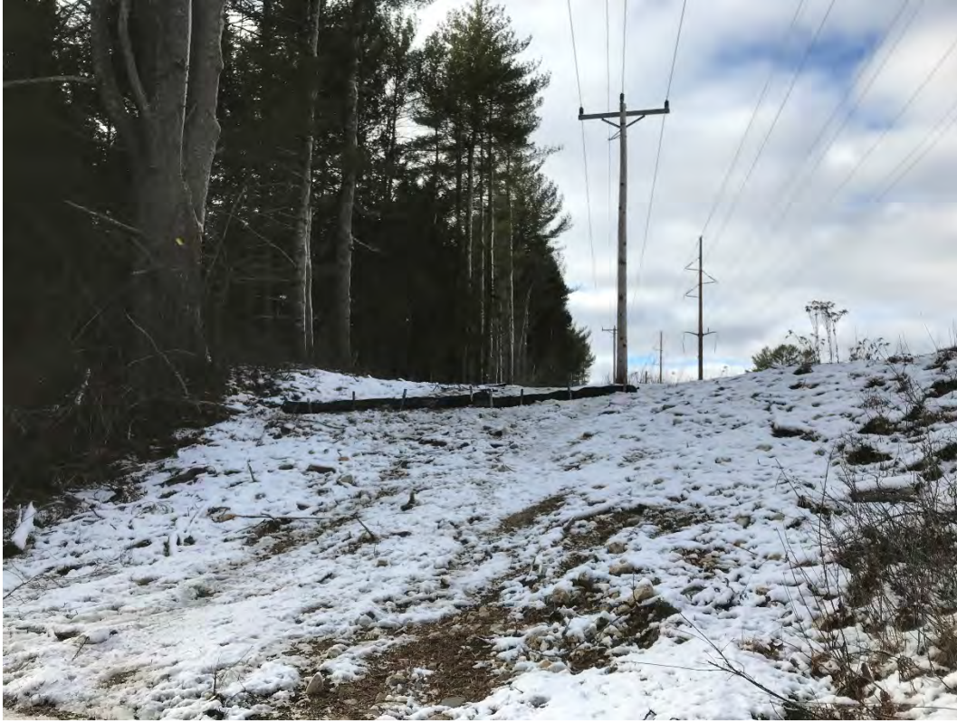
Fig 13: Line of silt sock installed on northeast facing slope above DS46 between Strs. 51 and 52. Viewing southwest. (12-07-20)
