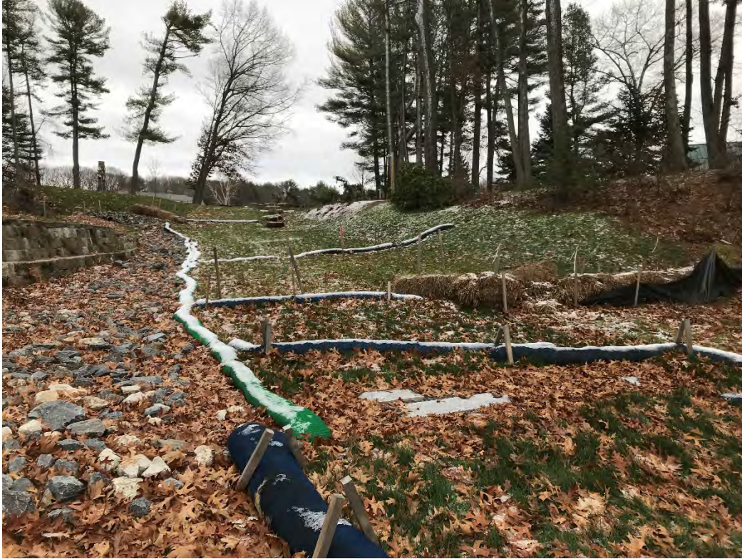
Fig 3: Slope above the manhole at Gundalow Landing/east side of the bay. Viewing east. (12-07-20)
