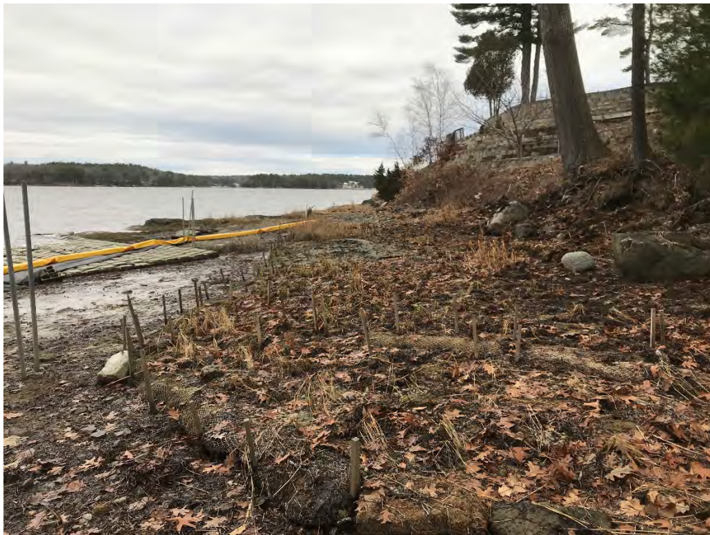
Fig 6: Salt marsh restoration at Gundalow Landing/east side of the bay. Viewing northwest. (12-07-20)
