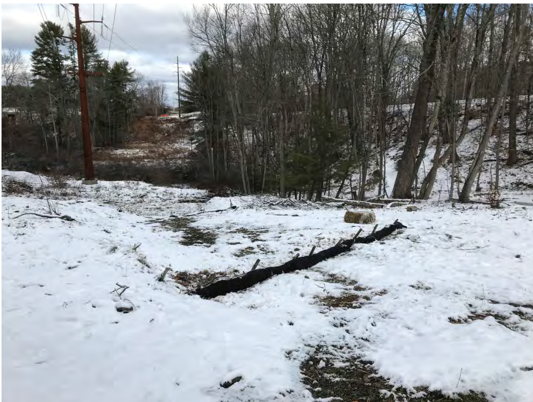
Fig 10: Additional line of silt socks installed on upper portion of slope between Strs. 28 and 29. Viewing northeast. (12-07-20)
